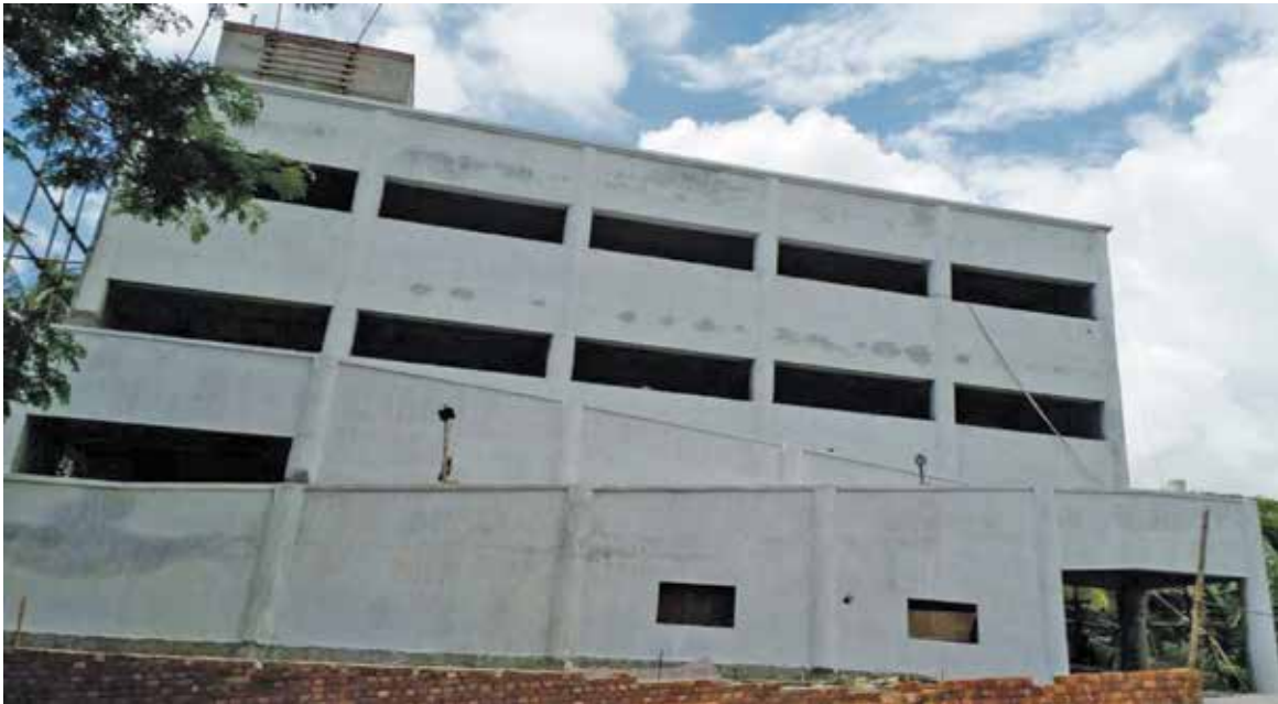
Construction of Cyclone Shelter under at Balisai Kanya Vidyalaya in East Medinipur District.
