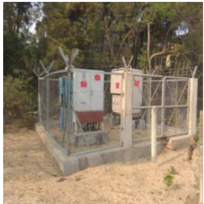
Underground Cabling Equipment, West Bengal
