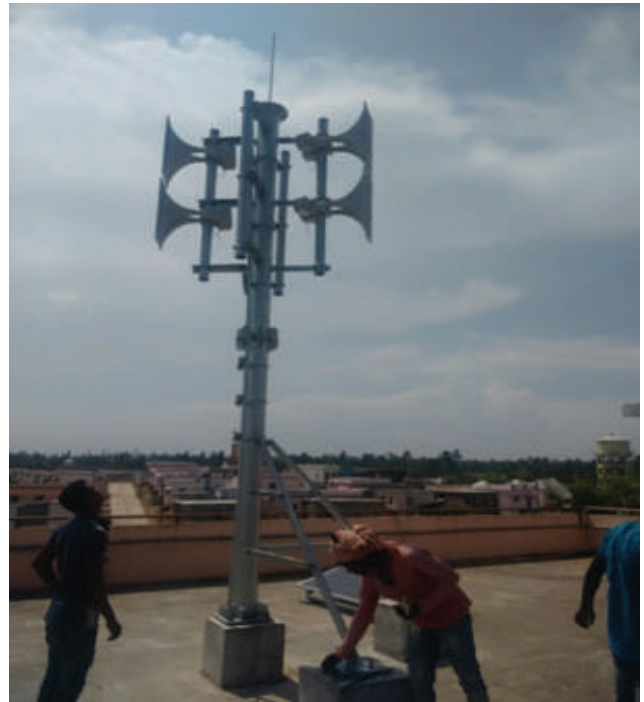
EWDS Monopole, Ganjam, Odisha
