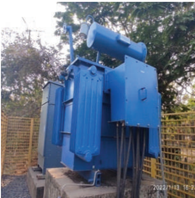
Underground Cabling Equipment, Goa
